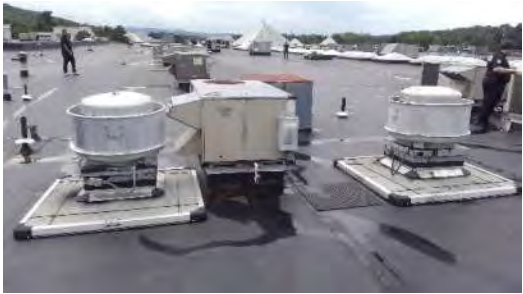
example of exhaust and plumbing vents located next to roof top unit intake
