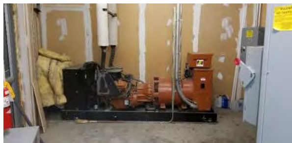
generator in electrical service #3 room
