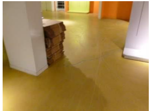
cracked concrete floor
