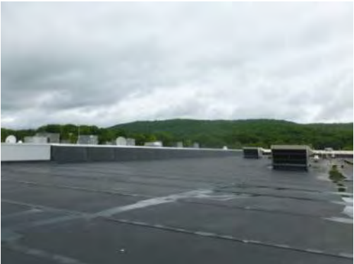
minimal ponding generally
