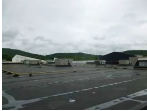
seam work/patching evident
