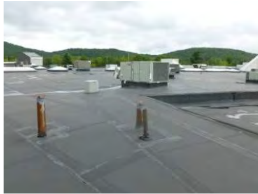
evident previous patching
