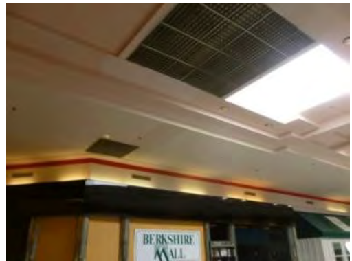
ceiling patches evident
