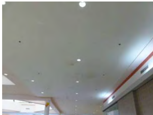
peeling and discolored ceiling finish
