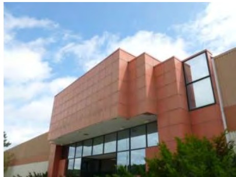
paneling at Sears; soffit damage
