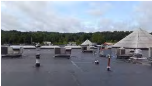
roof top units
