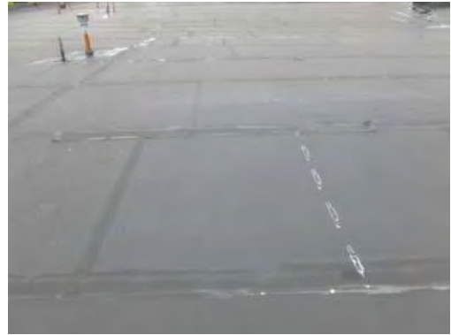
previous patches peeling up
