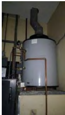
gas fired water heater
