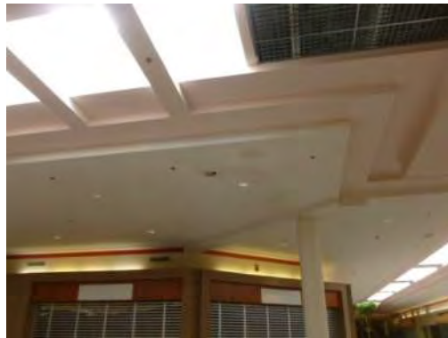
water stained ceiling
