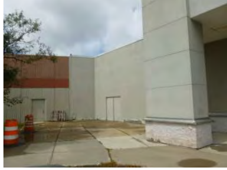
stained and damaged EIFS at Best Buy mall entrance
