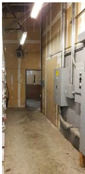
electrical service #3 room
