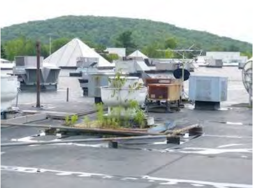
failing area of roof
