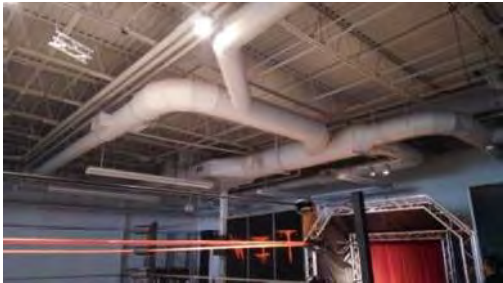
example of exposed ductwork
