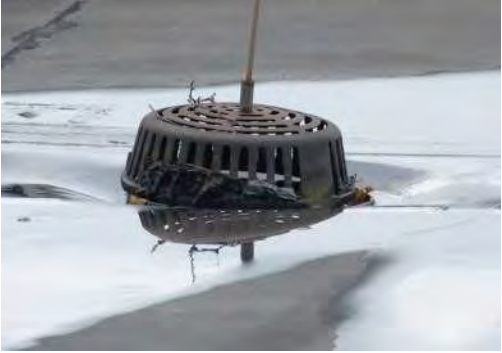
debris at drain
