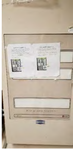
fire alarm control panel
