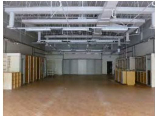
retail space – worn wood floor, open to structure
