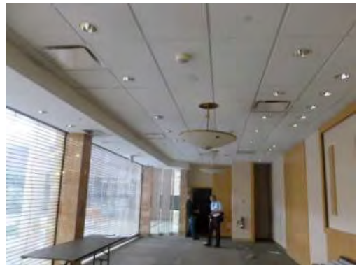
stained ceiling tile/carpet
