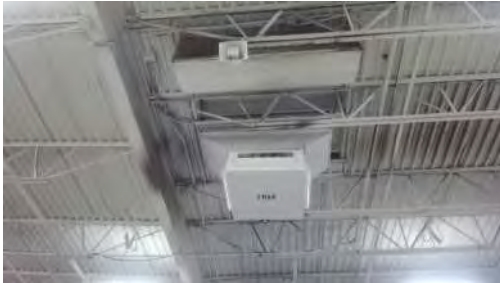
example of exposed ductwork
