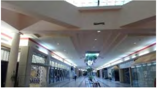
corridor supply grilles
