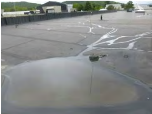
some ponding evident
