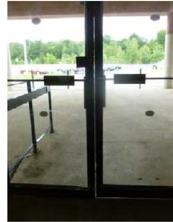
weather stripping absent
