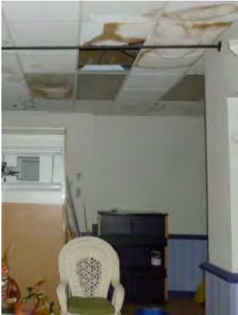
typical damage where suspended ceiling tile
