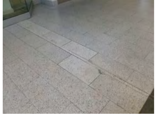
minor damage throughout to terrazzo
