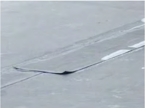
failing seam patch
