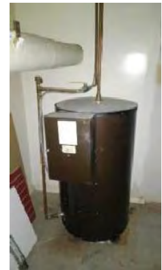
electric water heater
